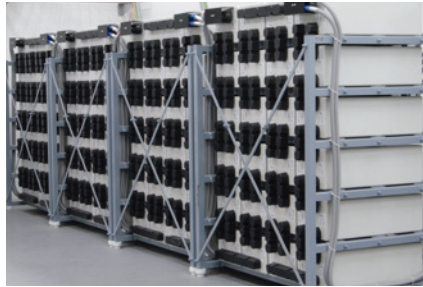
Energy Storage System
